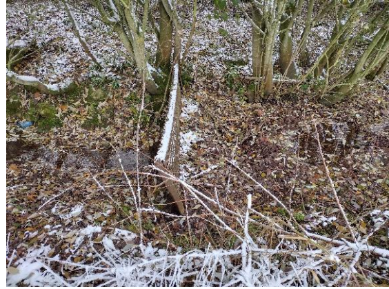
Figure 2.2 Grate crossing channel causing trapping of organic debris and backing up of water (looking from left bank to right at SP 52927 26132)
